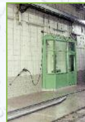
Hose trolley system.
