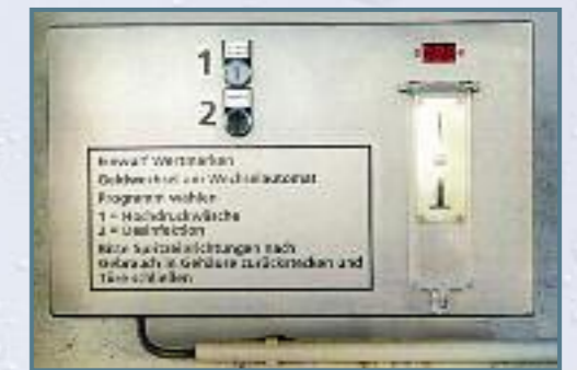
Remote control for a cleaning bay. This shows a customer tailored remote control for a slaughter house, cleaning and disinfecting of the trucks is here needed.
